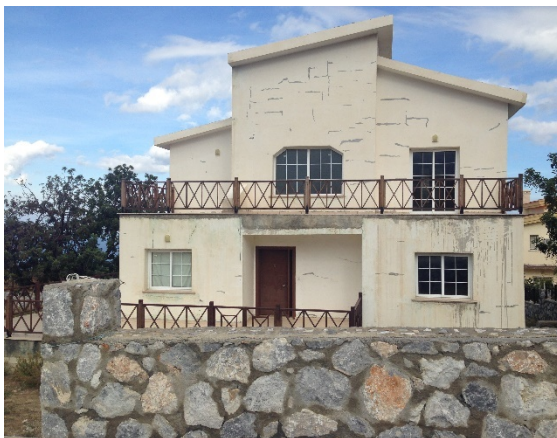
Figure 2. Biodiversity lost in housing and surrounding area built with reinforced concrete material (Take by author, Akansu, V., 2016)
