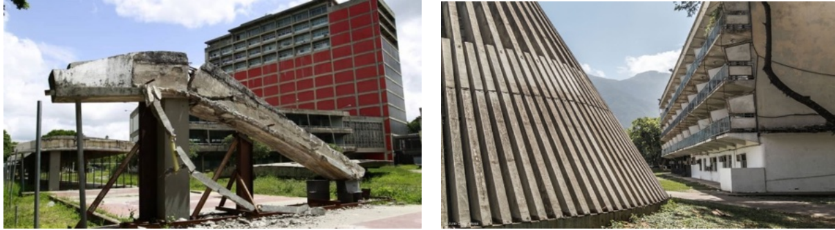
Figure 3. Some of the damages on the campus. /https://www.bbc.com/mundo/noticias-america-latina-58337209/
