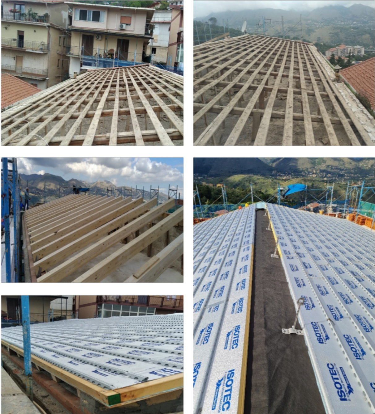
Figure 7. The rooftop structure before the intervention where it is possible to find the total absence of thermal devices as well as an under-sized structural elements; complete reconstruction of the new glulam beams, layer of insulation in monolithic rock wool panels and special integrated strip to allow the placement of the new tiles and central elements for the support of the ventilated ridge.
