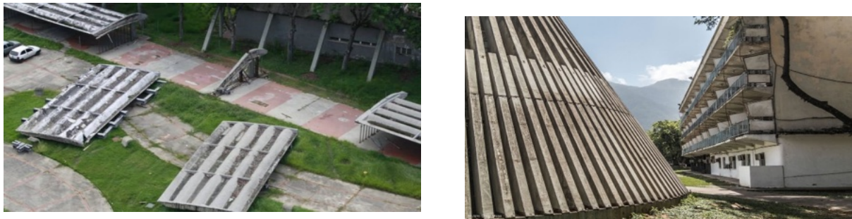
Figure 5. Some damaged fields that can be prioritized.
